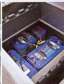
Batteries are neatly stored in their own compartment.
